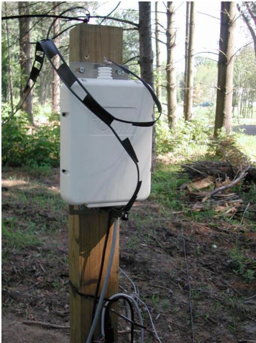
FIGURE 2: AH-4 IN OPERATION CONNECTED TO BALANCED ANTENNA
